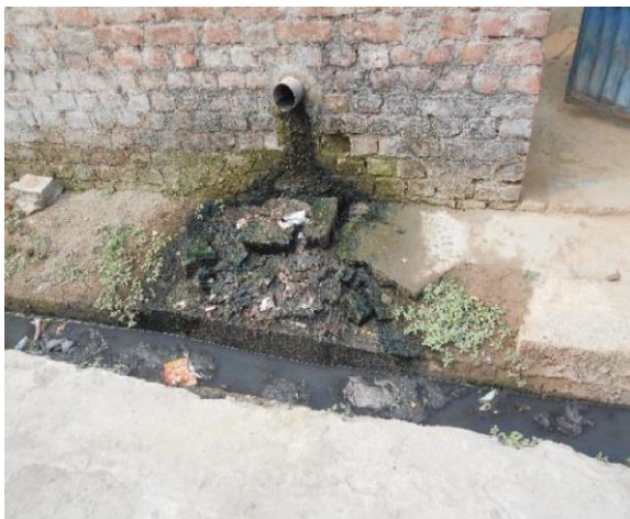
Black water from Septic tank
