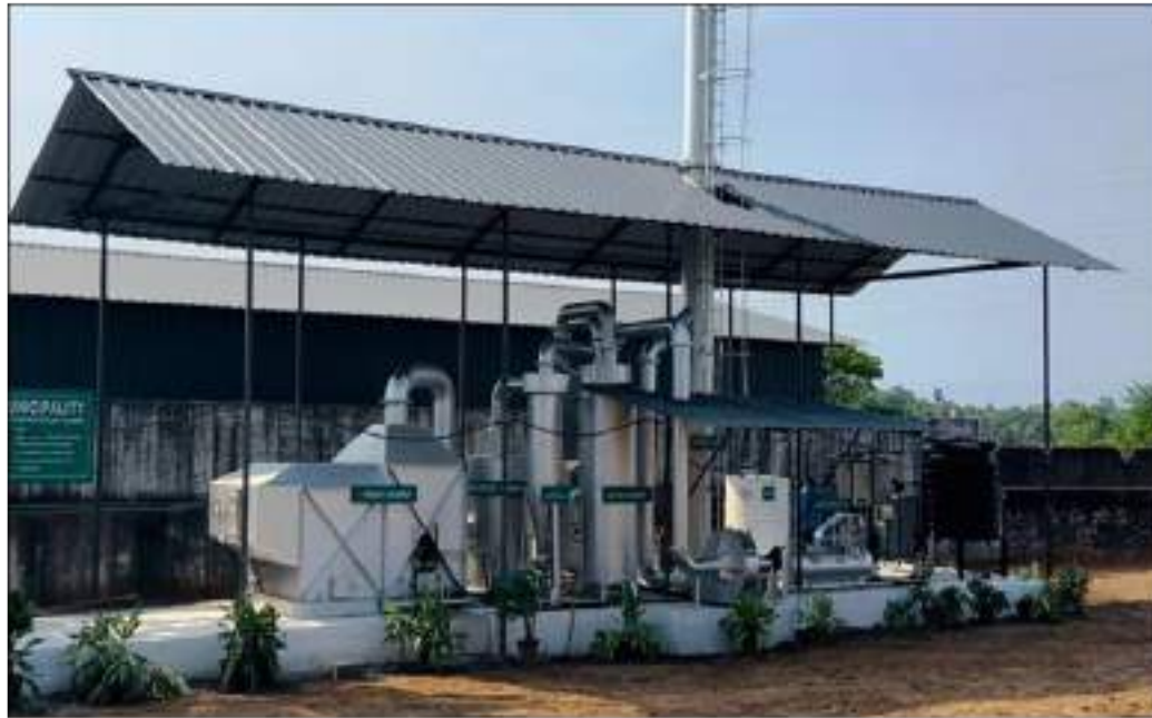
Double Chambered Incinerator at Palakkad Municipality.
