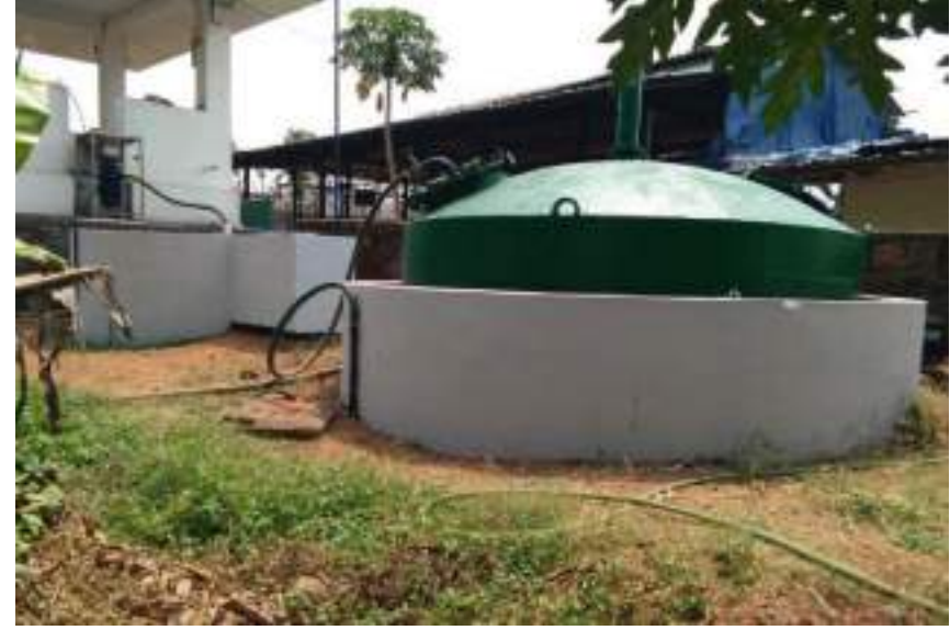
Floating Dome Biogas plant
